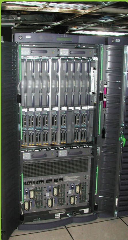
Storage/ Tape Backup Units
